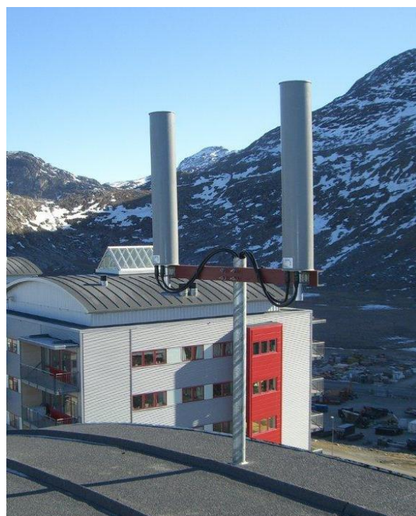
Figure 1 – Typical modern roof-top antenna system
